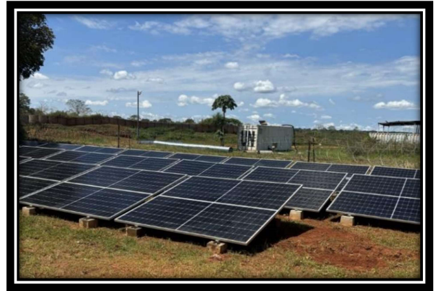
Pak Inf Batt in MINUSCA - Solar photovoltaic system low penetration system of 24 kWp deployed in 2023.
